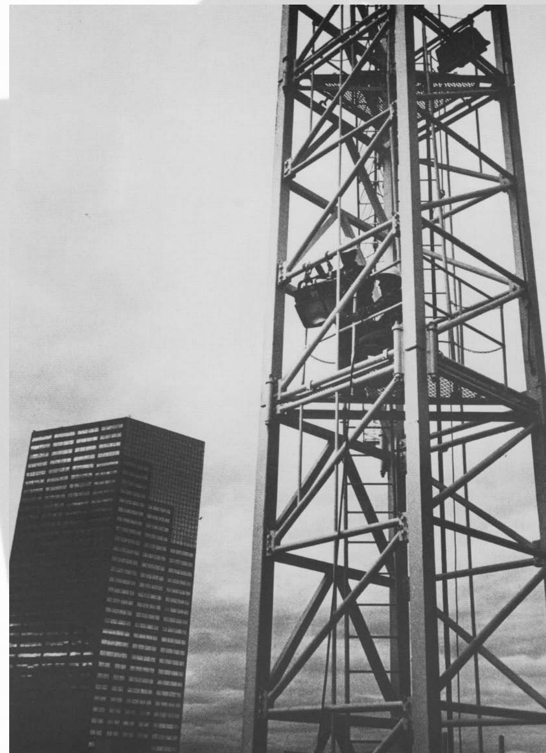
Ed Rasmussen and Tom Malloy of Christenson Electric install a crane light on Portland's One Oak Plaza building.
