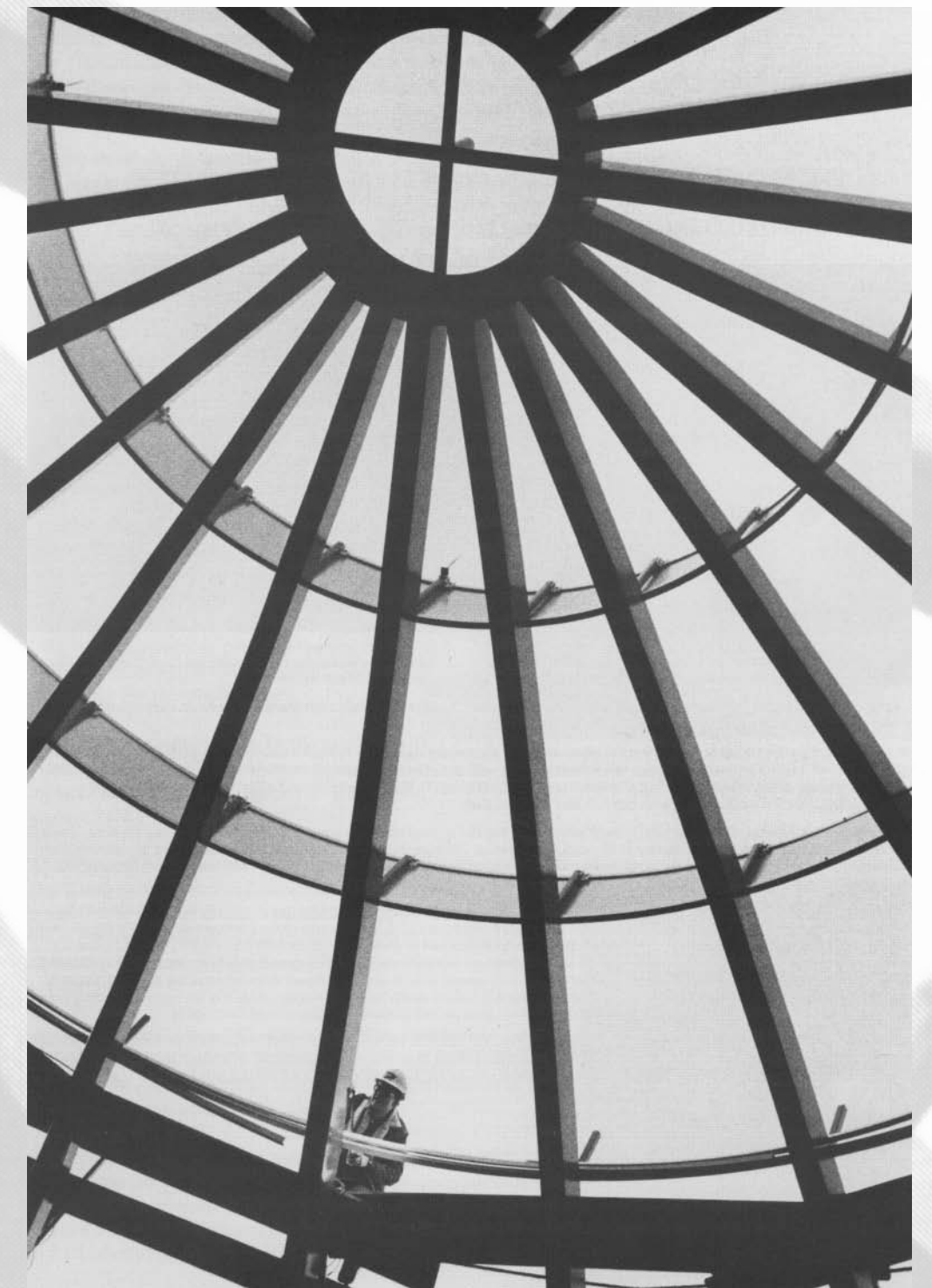
Christenson Electric's Ray Buschert installs a lighting rod atop the dome of Portland's 1000 Broadway tower.
